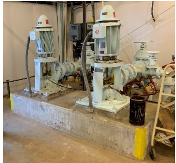
PHOTO 7.2.3 – FINISHED WATER PUMPS
