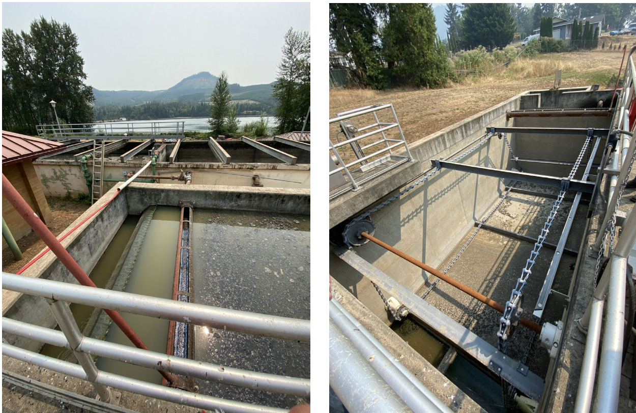
Figure 2-9: Primary Clarifier Weir and Scum Collector (Left) and Sludge Scraping Mechanism (Right)
