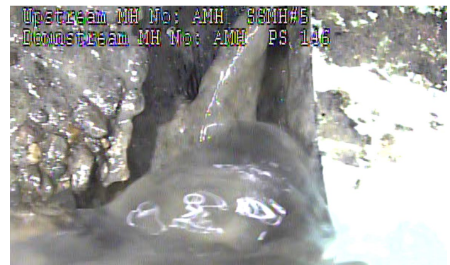
Figure 5: Broken Joint at Wet Well, From North
