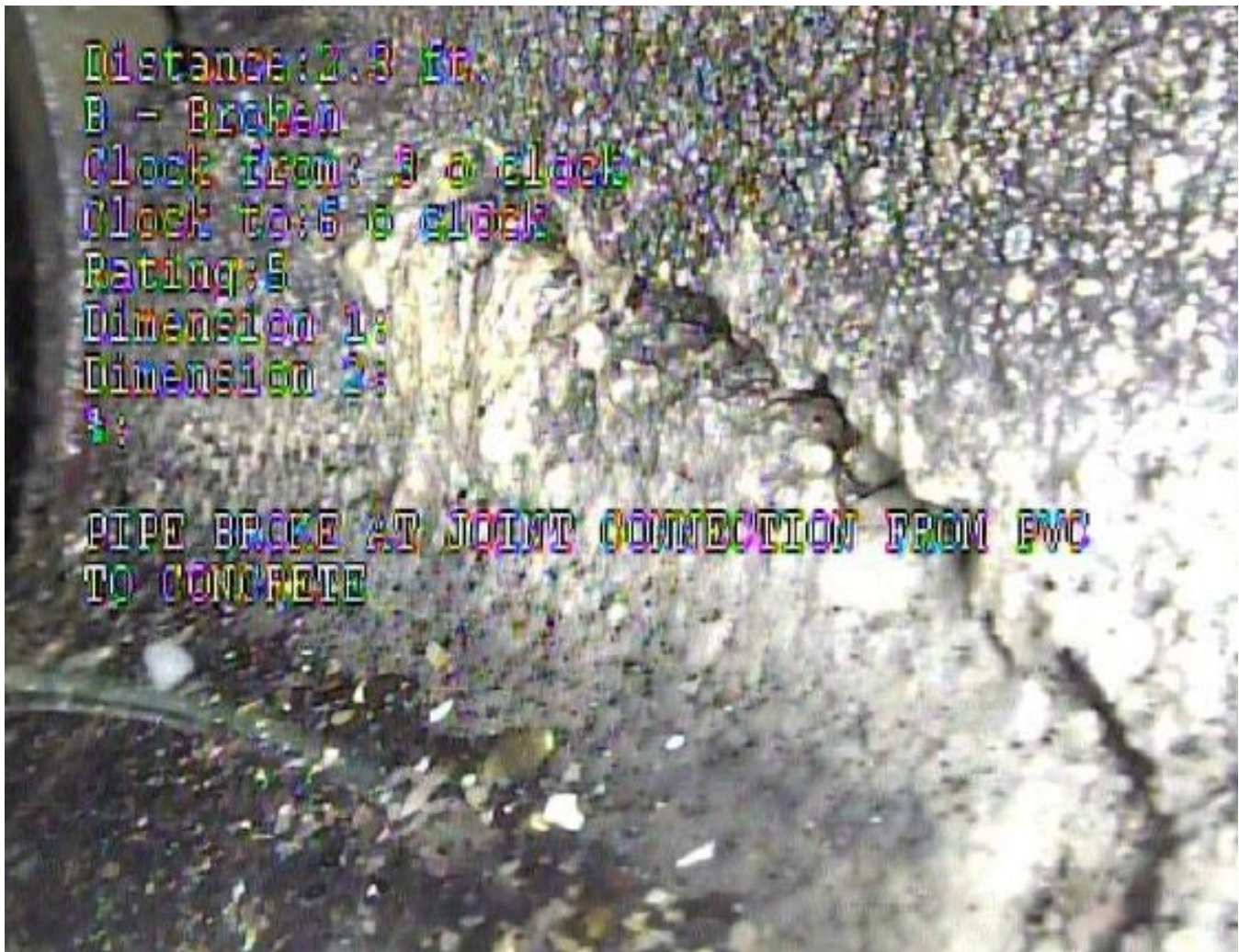
Figure 6: Broken Joint in Gravity Sewer under Rolling Rock Park
