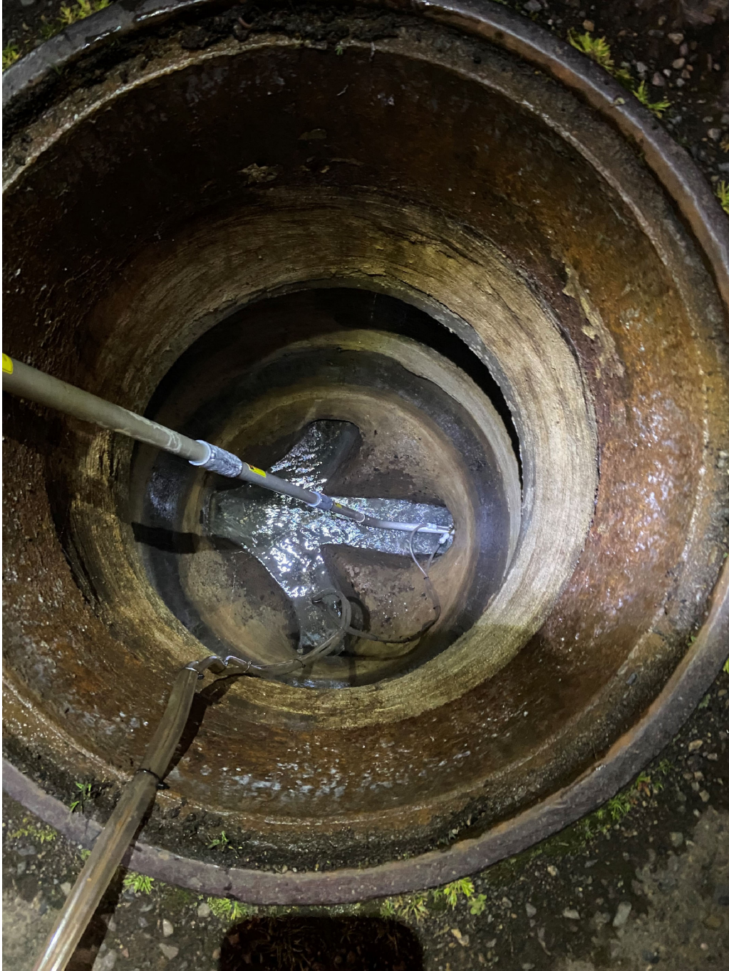
Manhole #57: Leak in grout between 1 st and 2 nd rings from bottom
