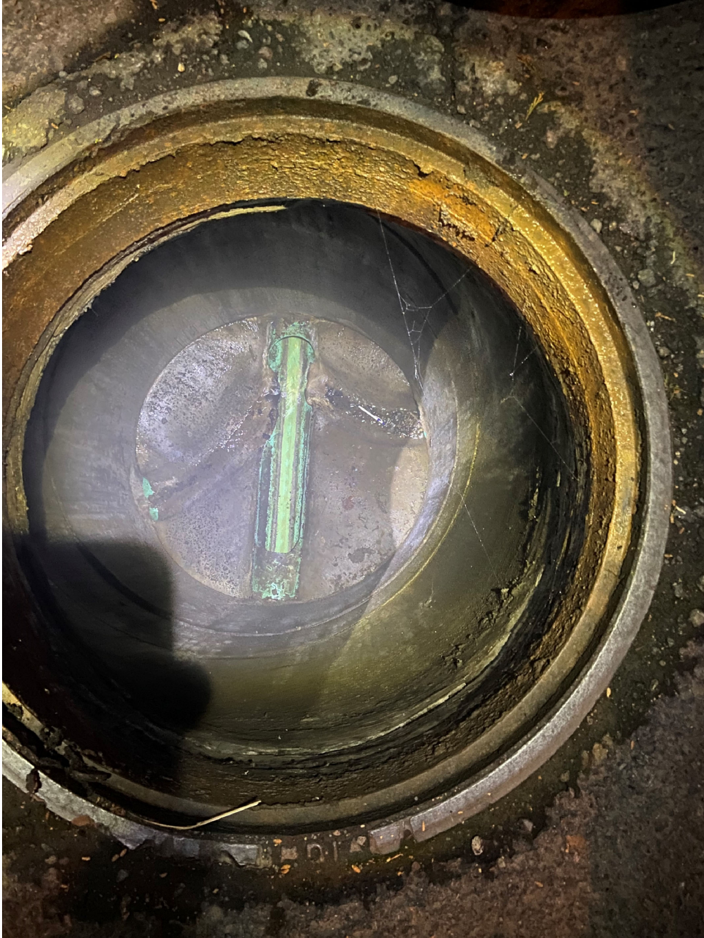
Manhole #68: Leak around circumference of outlet pipe
