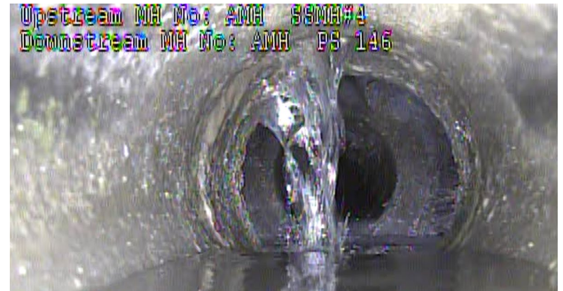
Figure 4: Broken Joint at Wet Well, From South
