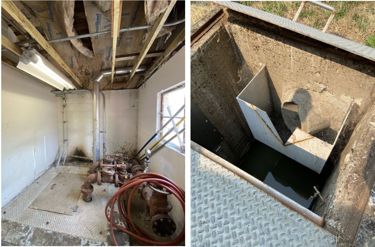
Figure 2-2: Alder Street Pump Station Wetwell and Intake (Left) and Emergency Overflow and Weir (Right)
