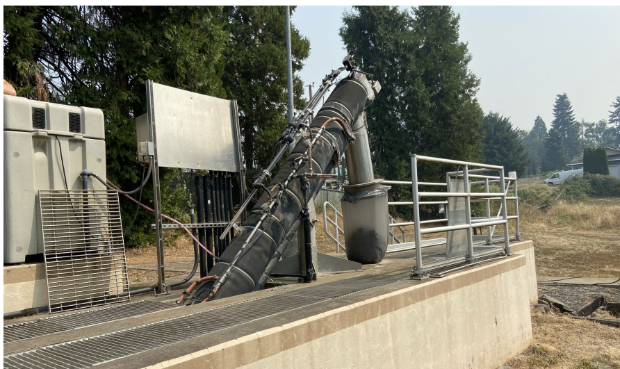
Figure 2-7: Inclined Fine Screen
