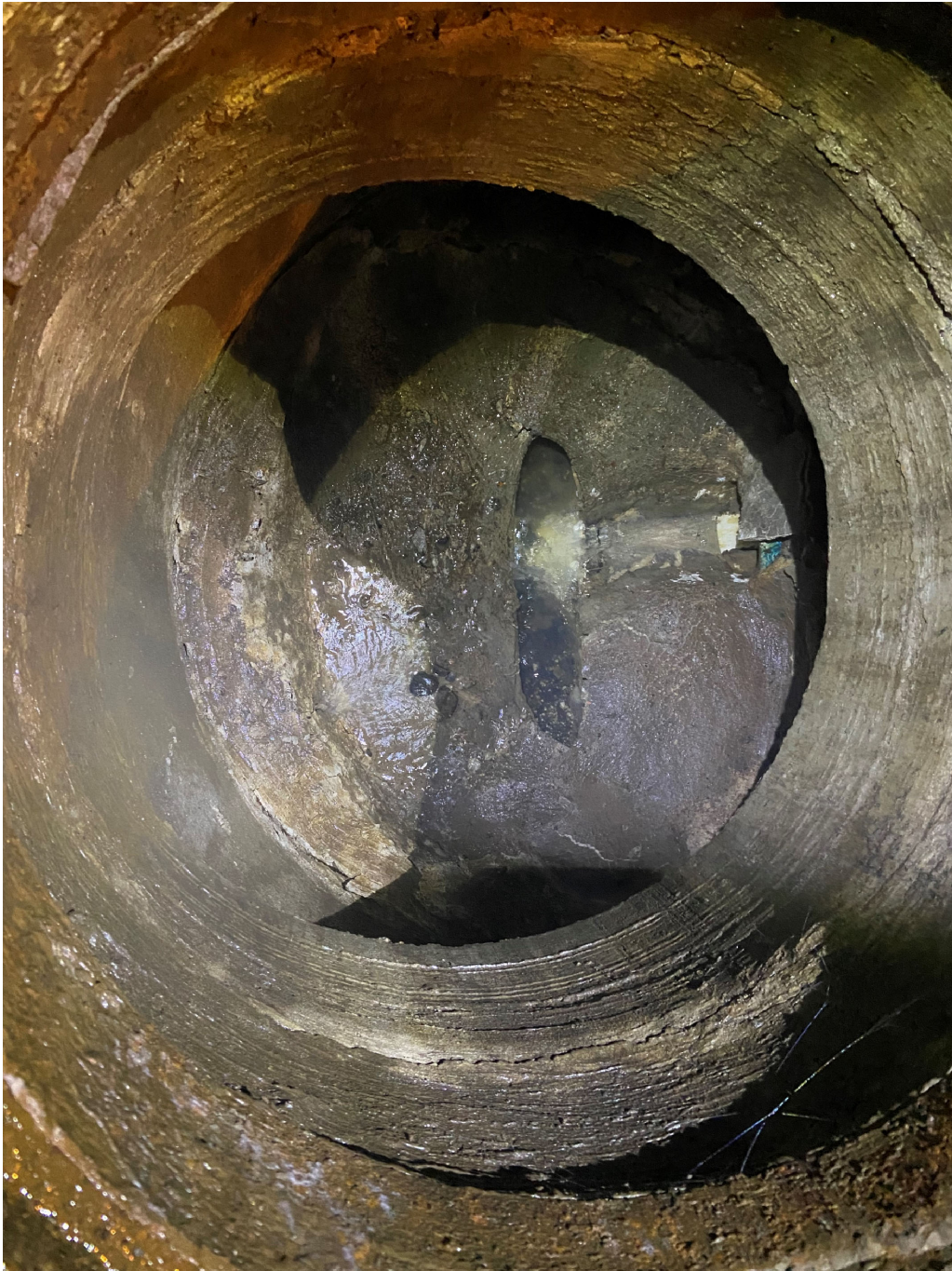
Manhole #79: Significant leaks in grout throughout entire manhole
