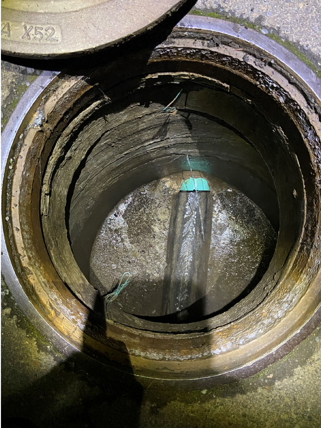
Manhole #80: Leak above inlet
