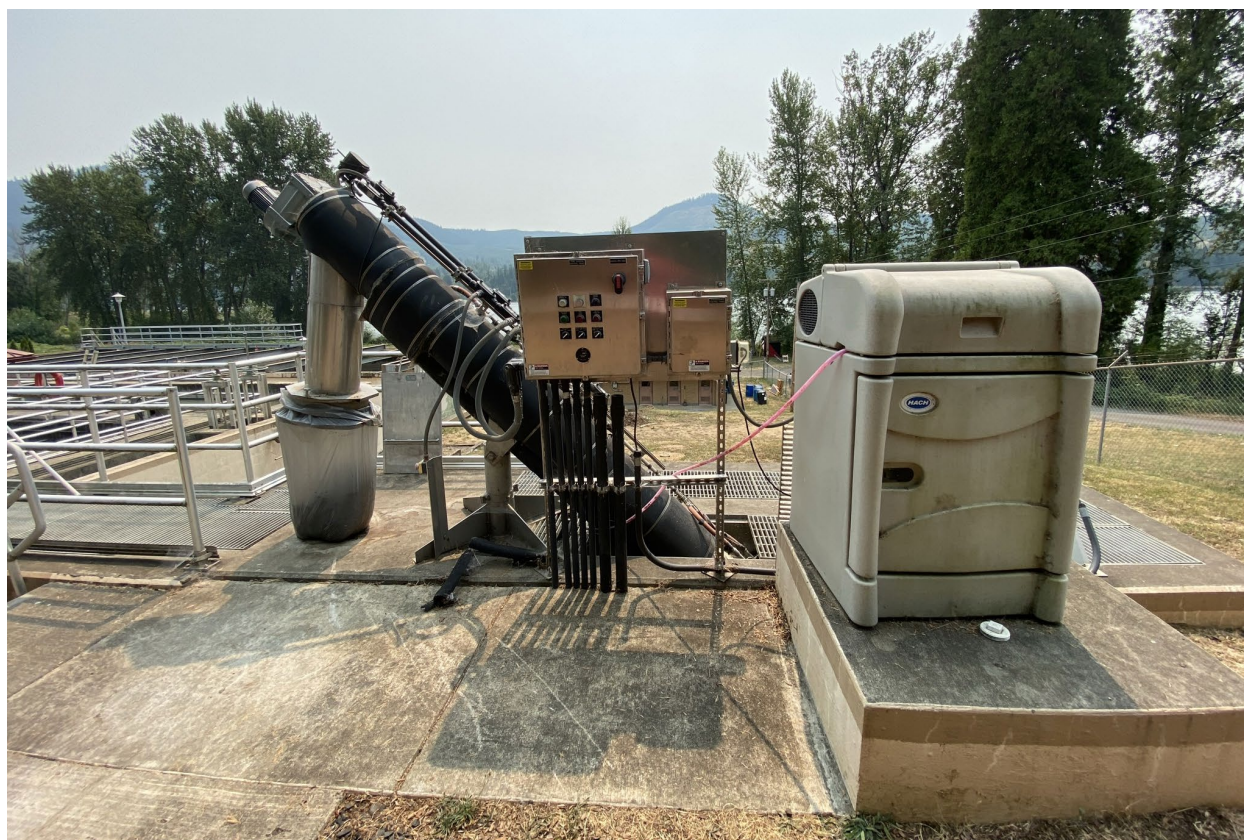
Figure 2-8: Influent Sampler and Fine Screen Control Panel
